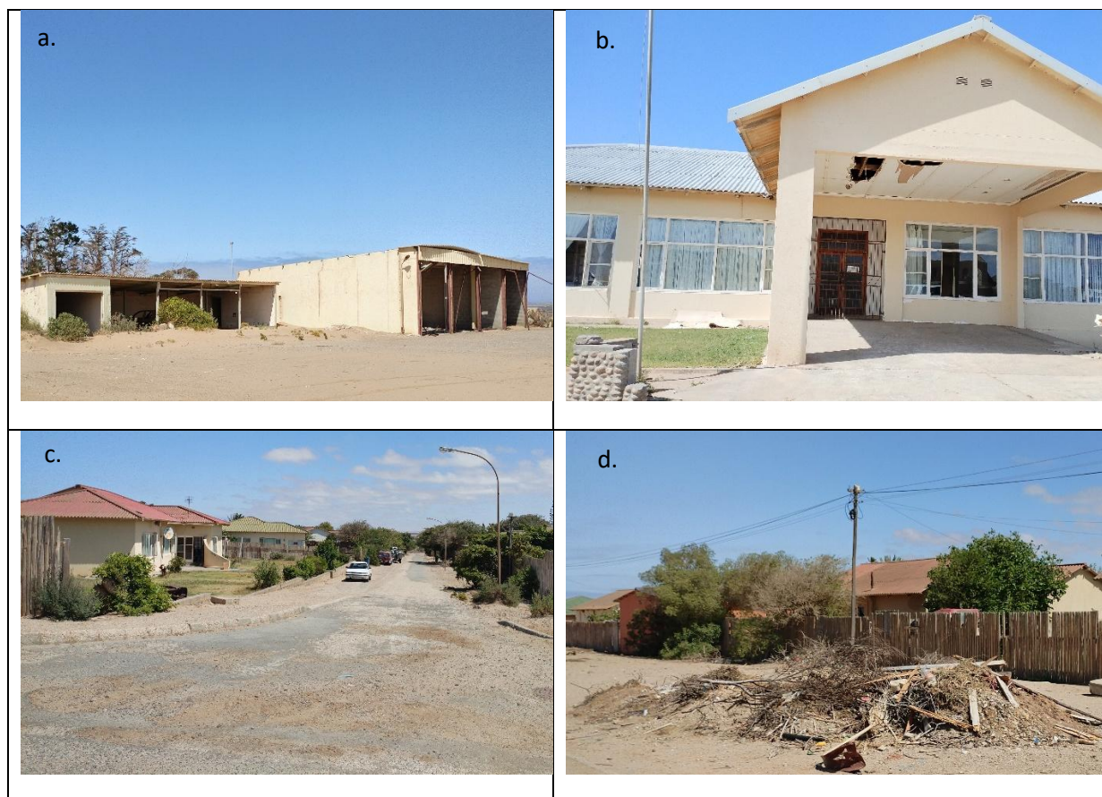
10 Figure 6-11: Alexander Bay: condition of infrastructure: a) Abandoned buildings, b) Damaged hospital, c) Decaying 11 streets, d) Rubble in streets.
