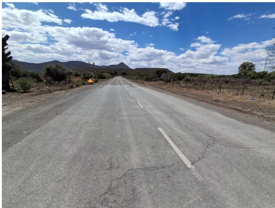
Figure B.5: Start of the MR00607 road in Murraysburg, showing the typical condition of the road (Source: CSIR, 2026)
