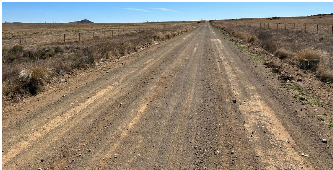
Figure 2.8: Photo of the S1262 taken along the gravel portion of the road (Source: Sturgeon Consulting, 2023).
