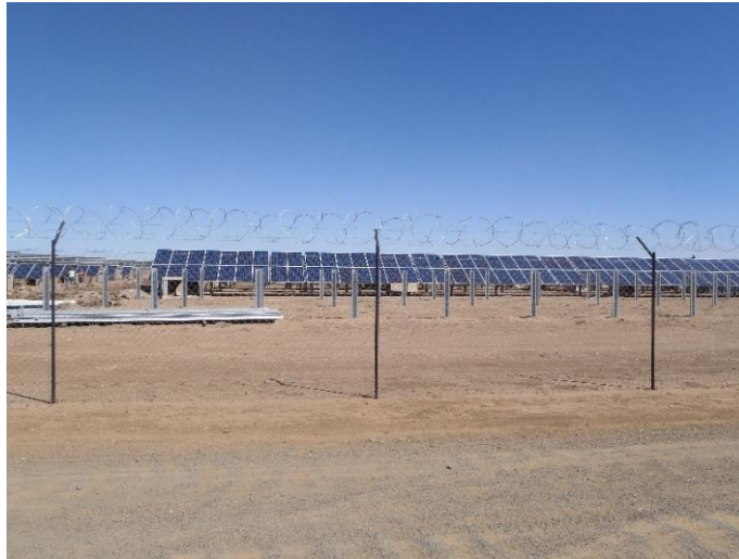
Figure A.6. Example of PV Technology (DFFE, 2019)
