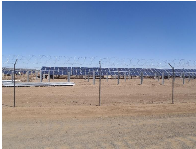
Figure A.6. Example of PV Technology (DFFE, 2019)
