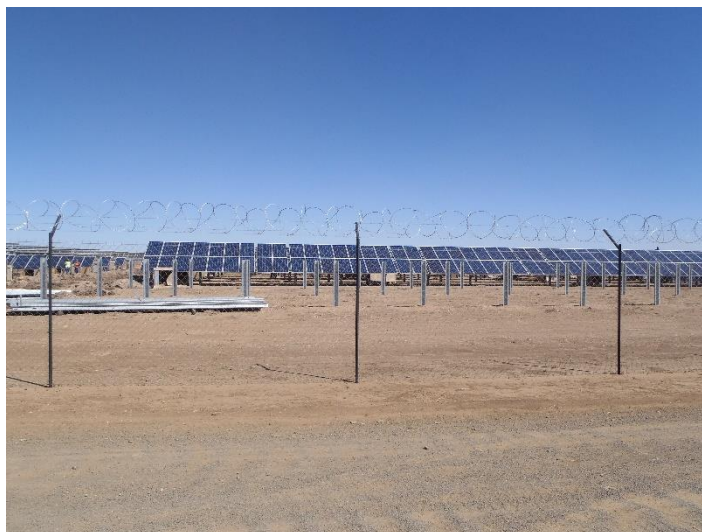
Figure A.8. Example of PV Technology (DEFF, 2019)
