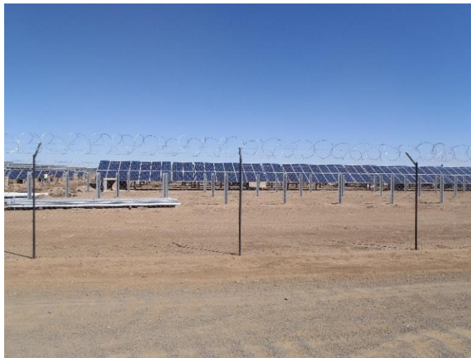
Figure A.6. Example of PV Technology (DFFE, 2019)
