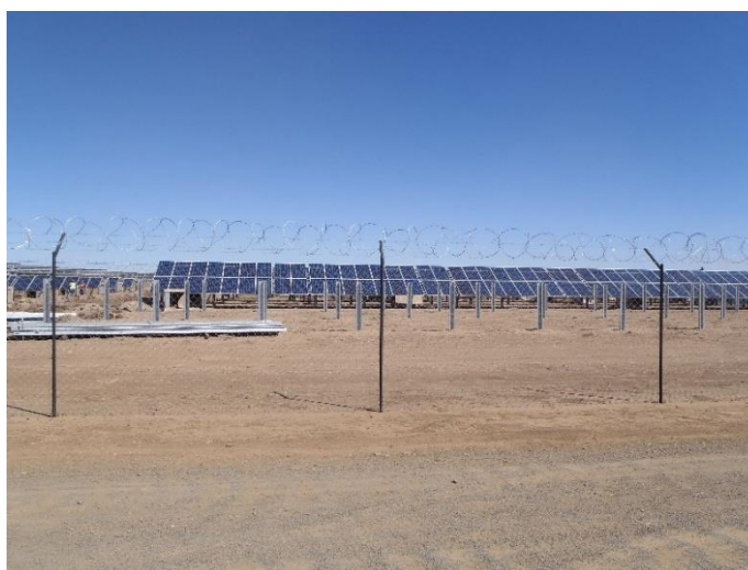
Figure A.6. Example of PV Technology (DFFE, 2019)
