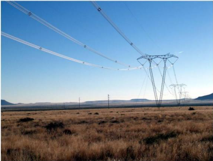
765kV Transmission Pylon @ 250m
