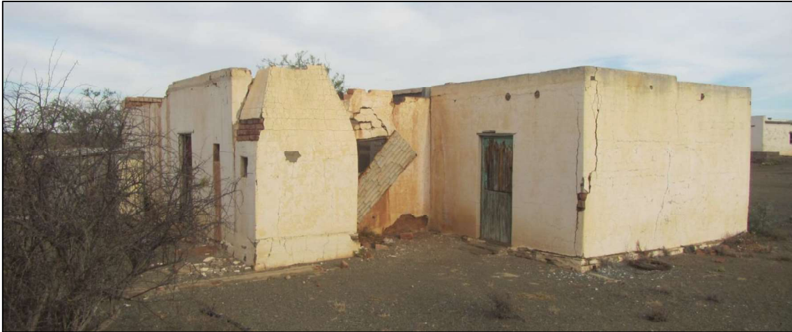
Figure 8: Example of a heritage resource of medium sensitivity (heritage grade IIIB). Although appearing in reasonable condition from the outside, the inside of this 19 th century house is in very poor shape due to its missing roof (waypoint 292).
