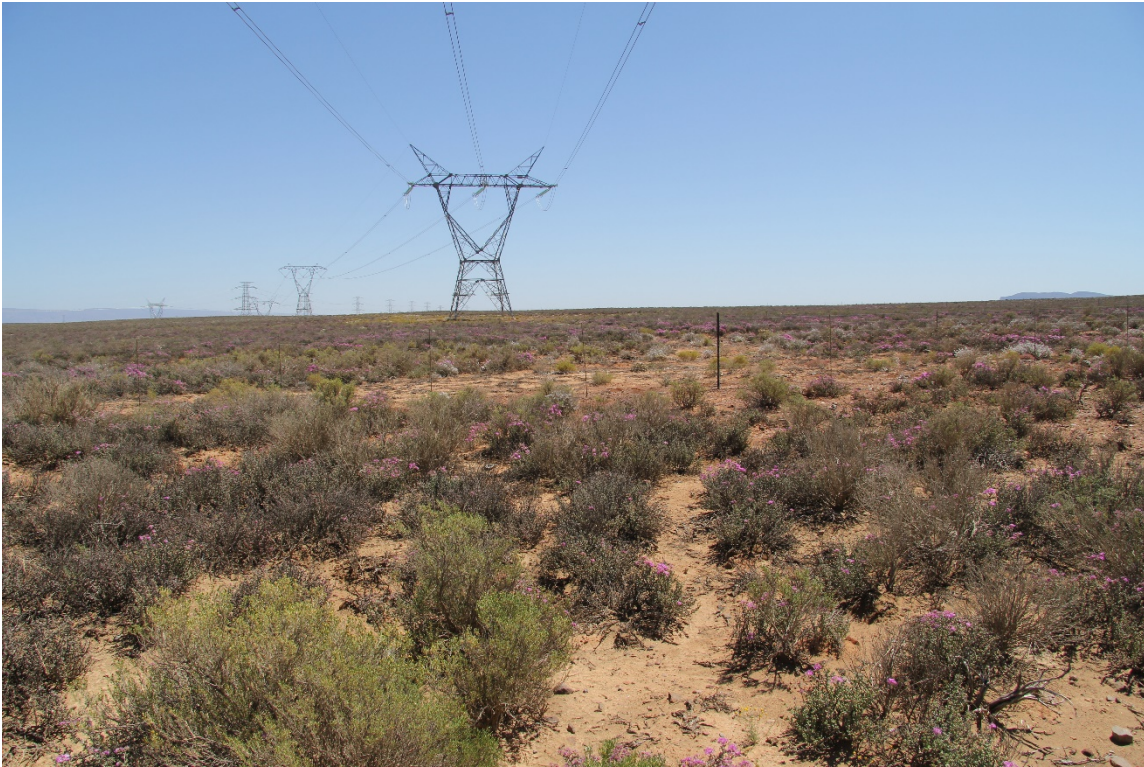
Figure 13: View of the power lines routed via the Eskom Kappa Substation on the Platfontein Farm (NW direction) (Photo: L. Kellerman)
