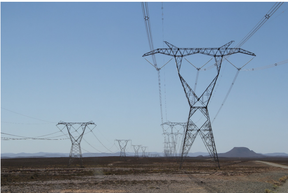
Figure 14: View of the power lines routed via the Eskom Kappa Substation on the Platfontein Farm (Photo: L. Kellerman)
