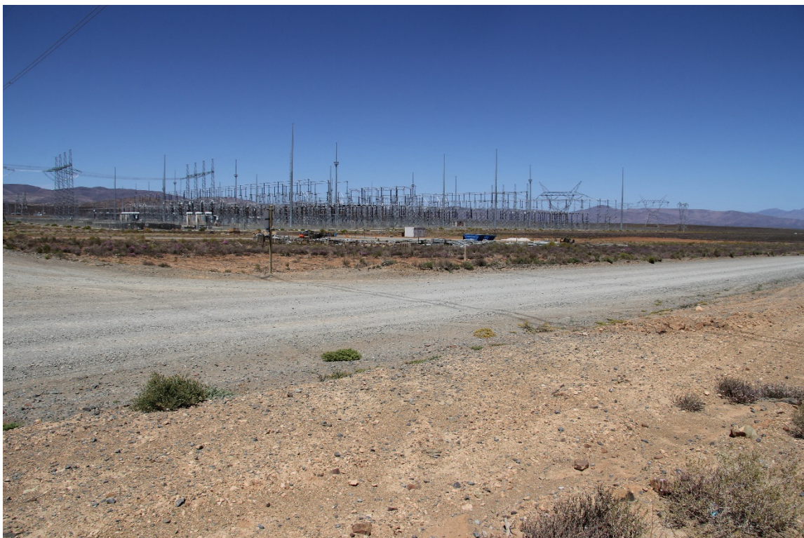
Figure 12: View of the northern side of the Eskom Kappa Substation on the Platfontein Farm (Photo: L. Kellerman)
