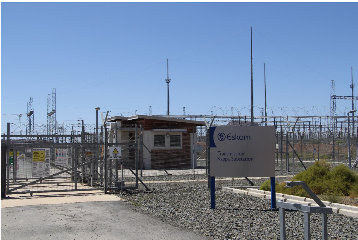
Figure 10: Official entrance to the Eskom Kappa Substation on the Platfontein Farm (Photo: L. Kellerman)
