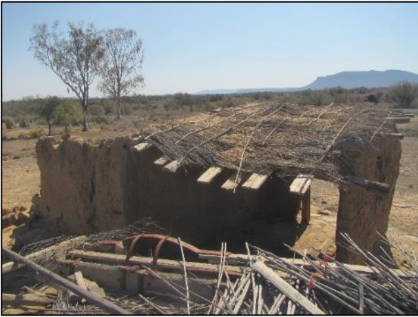
Figure 25: View of the roof of the ruin at waypoint 155. It was a brakdak.
