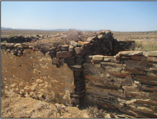
Figure 31: The join between the southern and central sections of the ruin at waypoint 158.
