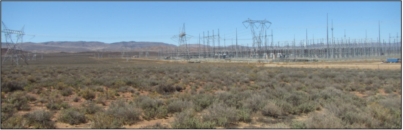
Figure 13: View towards the south of the Kappa Substation from within the southern end of the power line corridor. Photographed 28 January 2020.
