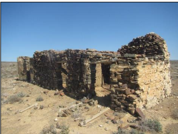
Figure 27: The front of the ruin at waypoint 158. The kitchen is at the near end.
