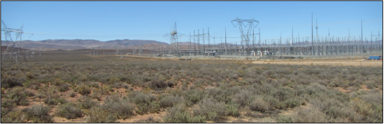
Figure 13: View towards the south of the Kappa Substation from within the southern end of the power line corridor. Photographed 28 January 2020.
