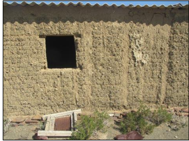
Figure 46: Wall detail showing weathered sun-dried bricks with the window frame having fallen out at waypoint 203.
