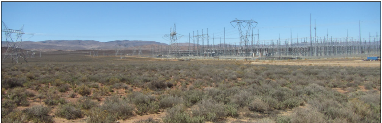
Figure 13: View towards the south of the Kappa Substation from within the southern end of the power line corridor. Photographed 28 January 2020.
