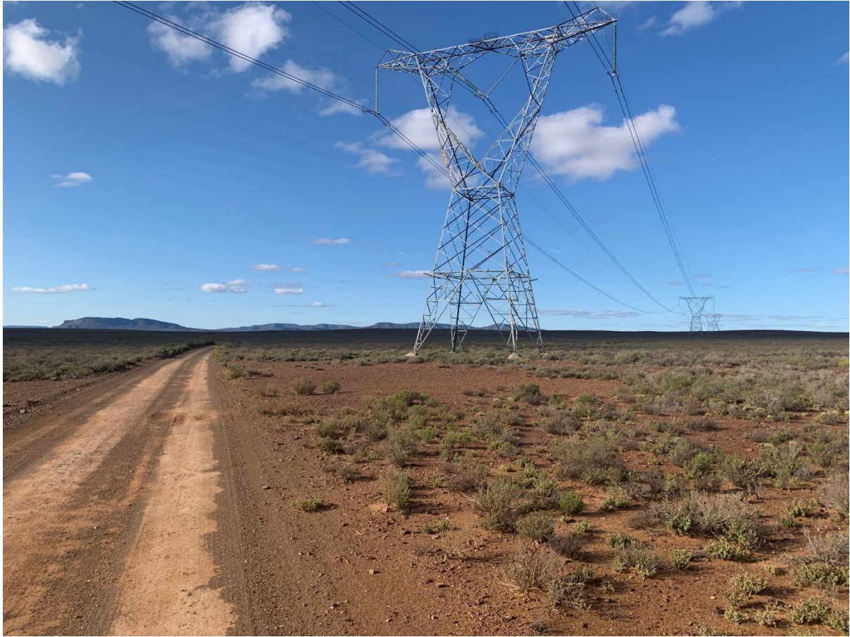
Figure 23. Image showing nature of the corridor to be traversed by the electrical powerlines serving the Kappa substation and existing powerlines proximal to the servitude on the Farm Die Brak.
