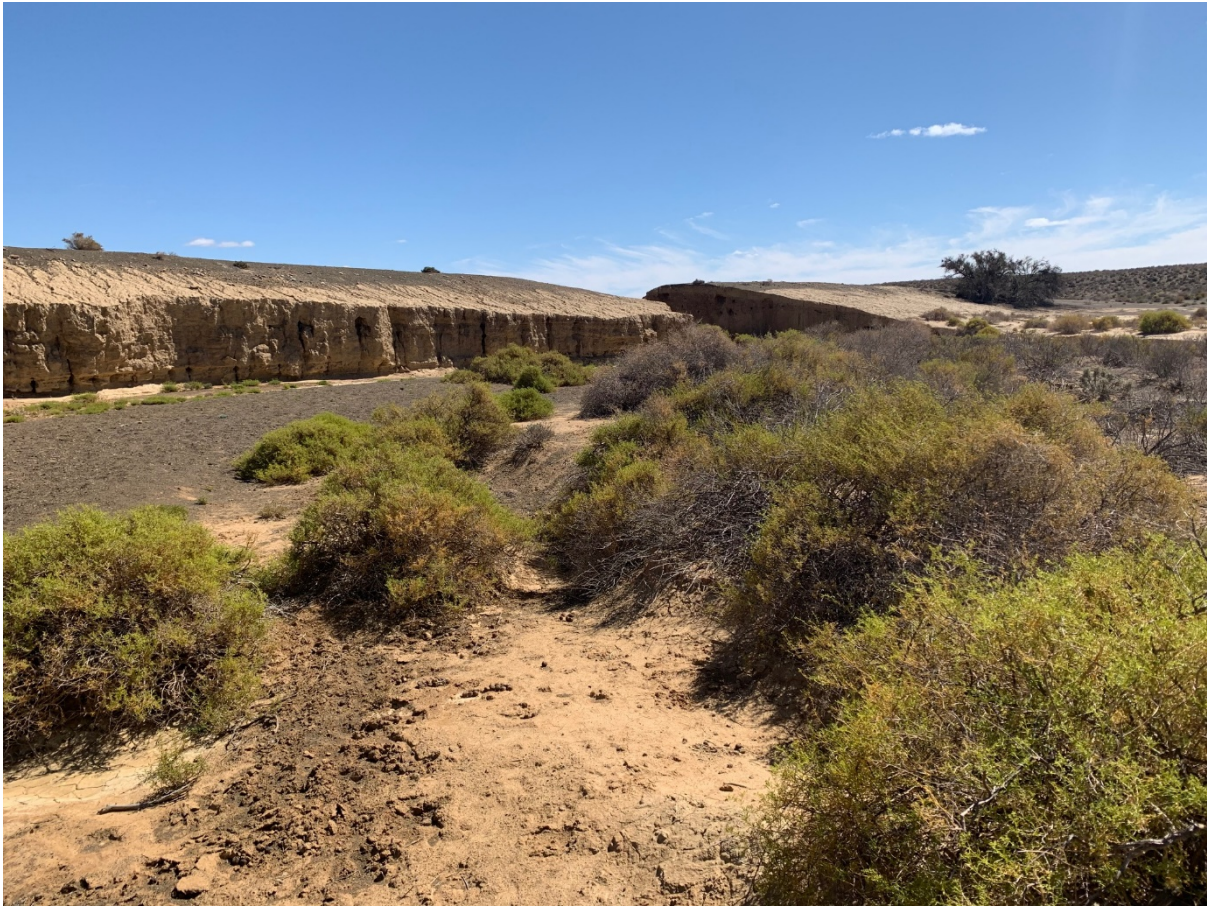
Figure 6. Image of the dam wall within the Hoek Doornen farm area – note breach within the centre of the wall.
