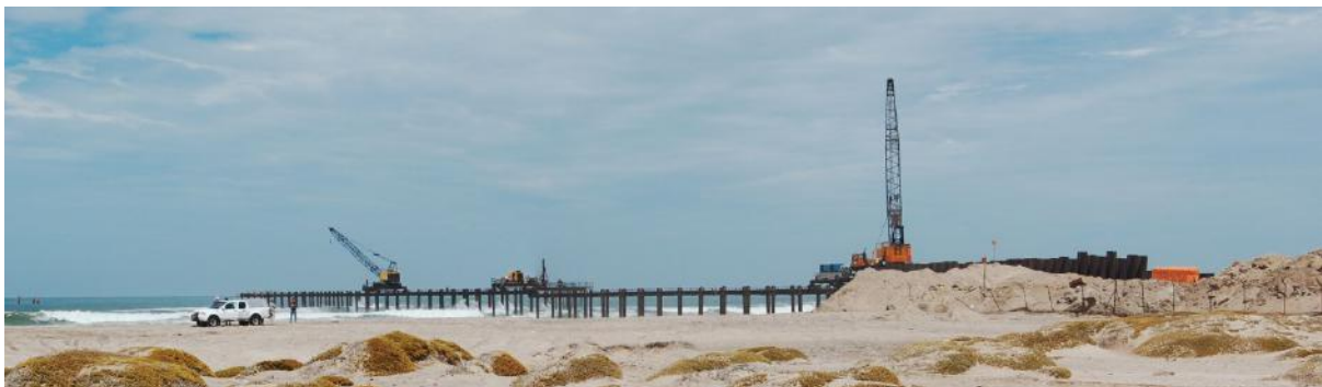
Figure 10-51 Example of a construction jetty at the desalination plant at Wlotzkasbaken, Namibia.
