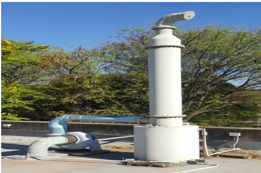
Scrubber on roof above laboratory
