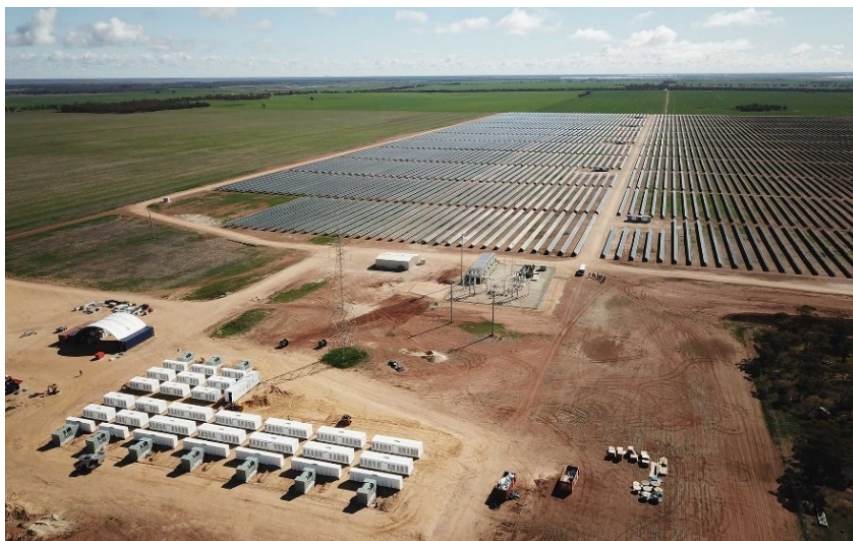
Figure 2.5. Example of PV Technology with Lithium Ion BESS (ARENAWIRE, 2018 2 )
