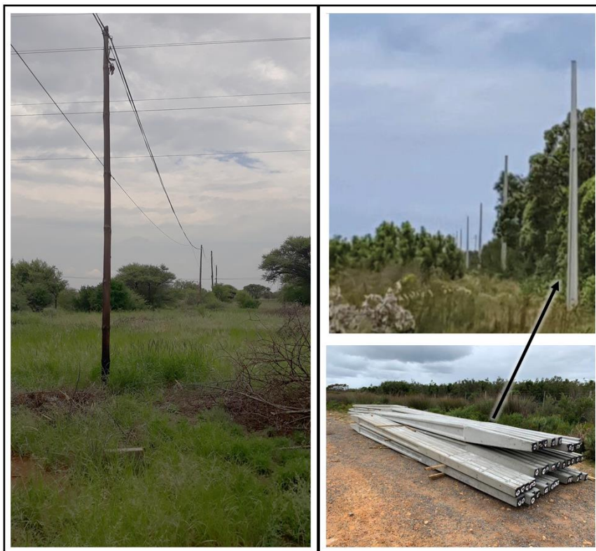
Figure 6: Examples of fibre optic cables installed on timber (left) and concrete (right) poles.
