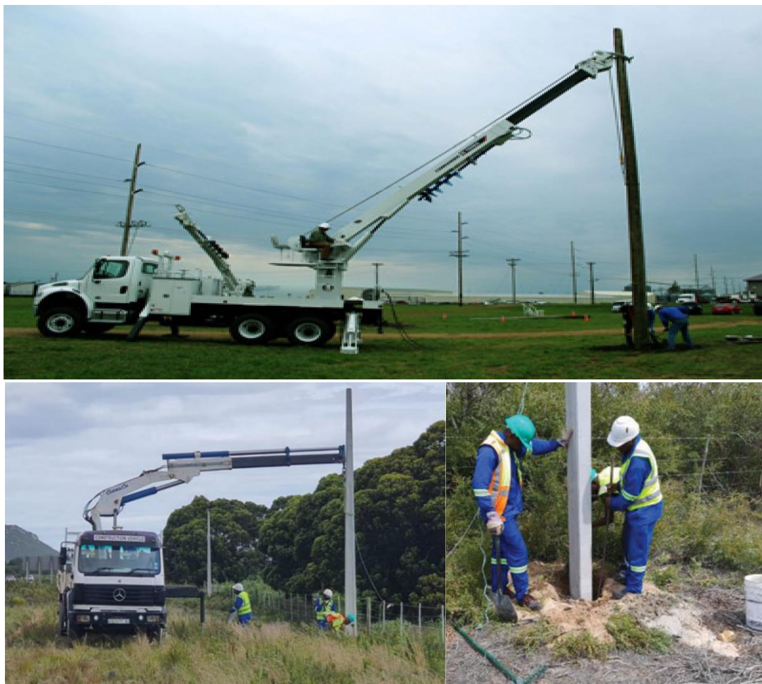
Figure 8: Example of a truck used to plant timber (top) and concrete (bottom) poles.
