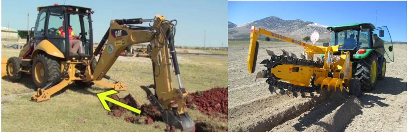
Figure 3: Example of machinery used to dig trenches -Tractor Loader Backhoe (TLB) (left) and Chain Trencher (right).
