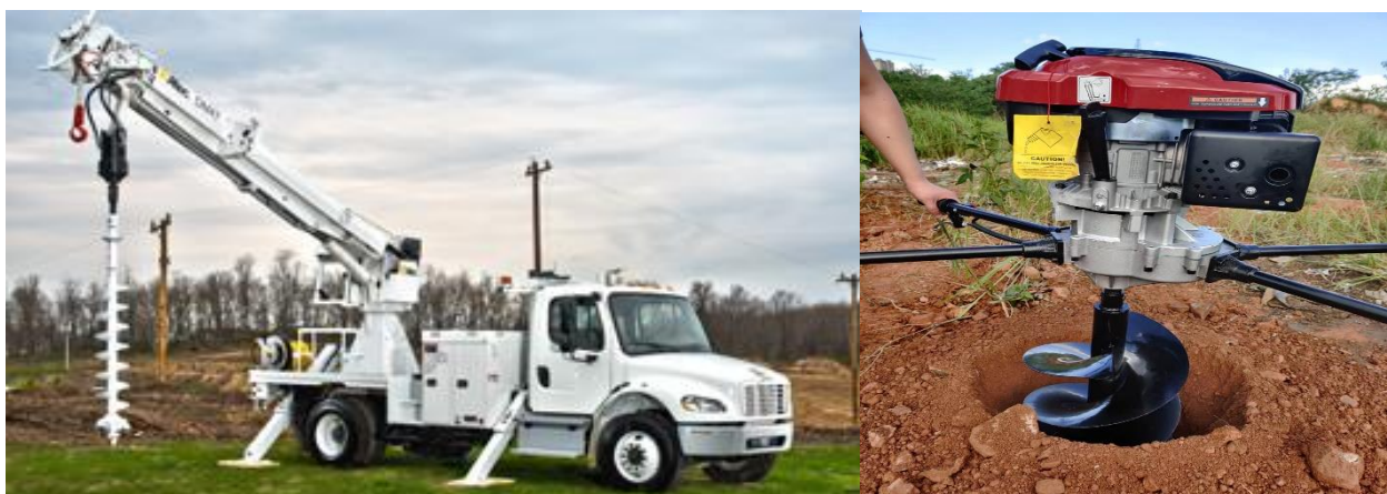
Figure 8: Holes for installing overhead cabling poles will be dug by truck-mounted (left) or hand-held (right) drills.
