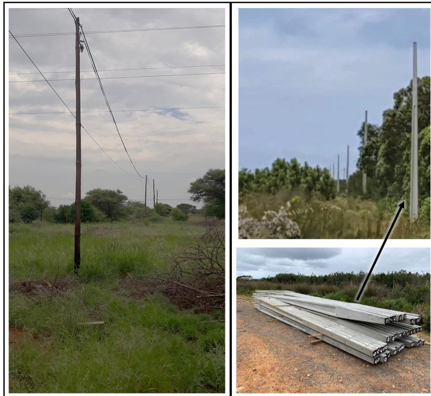
Figure 7: Examples of fibre optic cables installed on timber (left) and concrete (right) poles.
