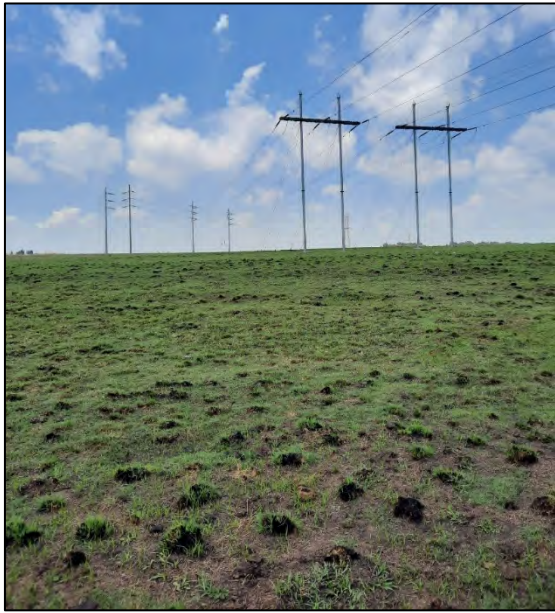
Figure 3-56: Grass cover and powerlines.
