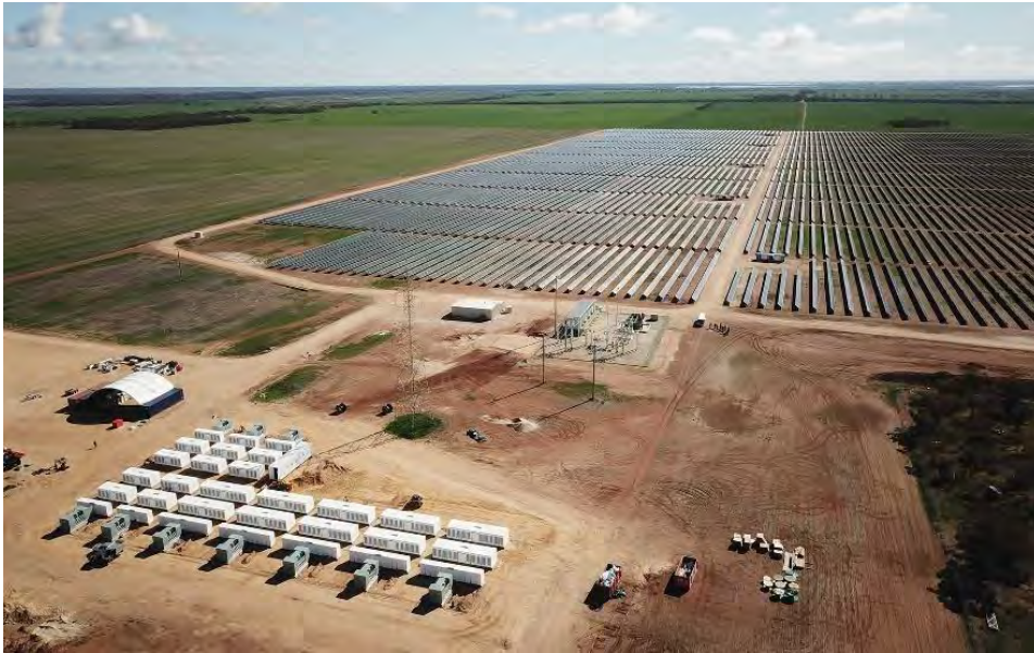
Figure 2-3: Example of PV Technology with Lithium-Ion BESS (ARENAWIRE, 2018 1 )
